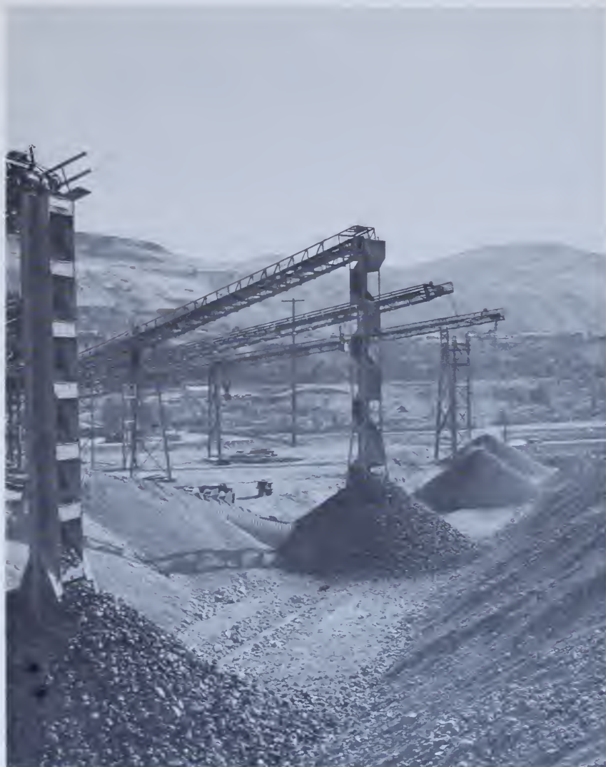
Figure 82. —Rock ladders used at Grand Coulee Third Powerplant in Washington. These effectively reduce breakage of coarse aggregate. P1222-142-10039.
